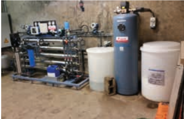
— The new reverse osmosis installation. Photo Wim Speliers.
